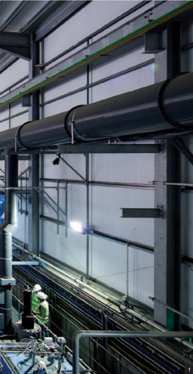
1. This state-of-the-art anaerobic digestion plant in Cannock, Staffordshire is the biggest in the UK. The facility processes up to 120,000 tonnes of food waste from homes and businesses every year to produce both enough renewable energy to power 6,000 homes and a soil improver that can be used in the same way as compost. The process uses naturally occurring micro-organisms already present in food waste to break it down in the absence of oxygen. The waste reception area of the main building operates under negative air pressure to prevent the escape of odour and dust and the process takes place entirely within a closed environment. Rapid open/shut doors maintain negative air pressure while waste is delivered and compost removed.
